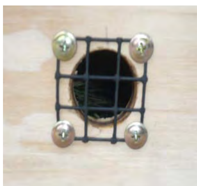
Figure 7: Close up of ventilation holes covered with 10mm aviary mesh. (K. Elliott, 2009).
